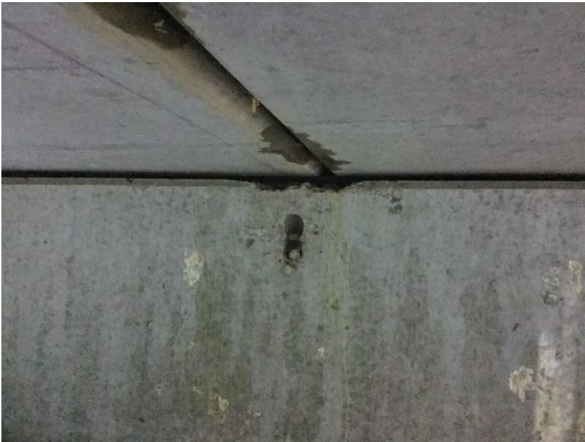
Minor cap spalls
